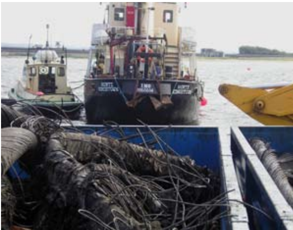
After being lifted from the ocean bottom the old ocean cables are shortened with LUKAS cutters so that they can be loaded for transport in containers.
